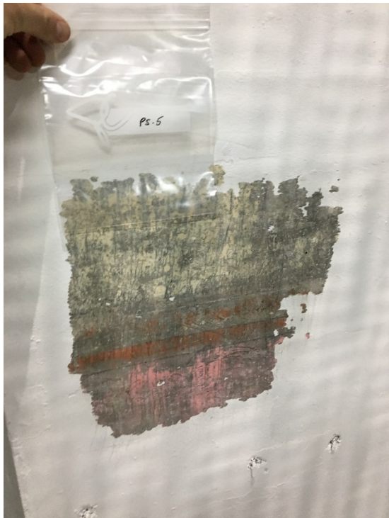
Photo 6 Paint sample PS-5 and sampling area. Concrete wall in CT3 BOP area basement.
