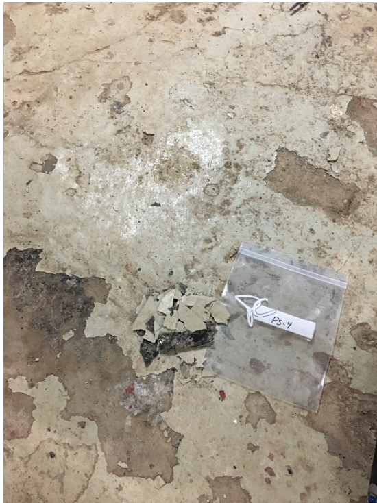
Photo 5 Paint sample PS-4 and sampling area. Concrete floor in CT3 BOP area basement.
