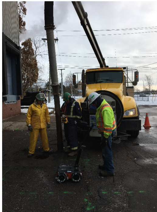
Photo 2 RL Dennis using ground penetrating radar to mark out utilities in the ground prior to hydroexcavating MW-4, looking southeast.
