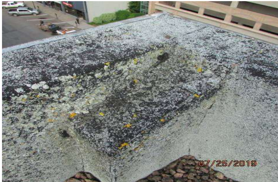
Severe granule loss on base flashing membrane.
