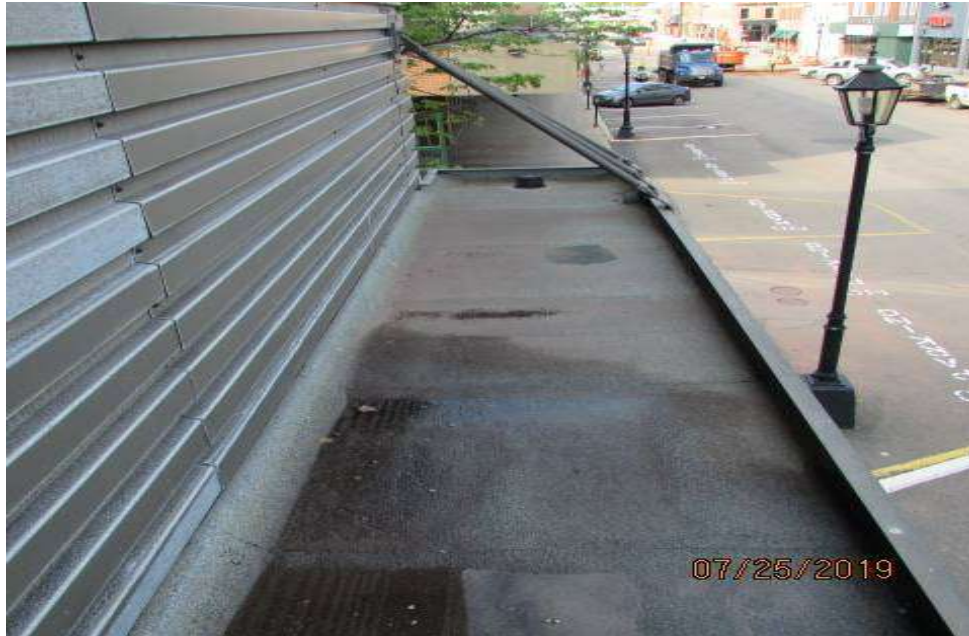
View of roof. Drain is located in high location of roof decking on south side of building.
