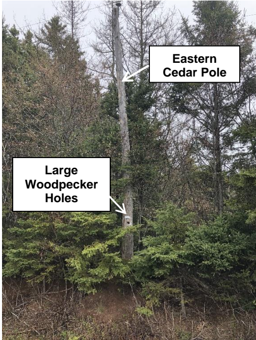
Damaged Pole (reduced pole strength)
