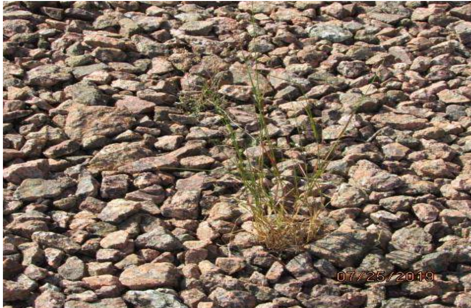
Vegetation growth on roof surface,
