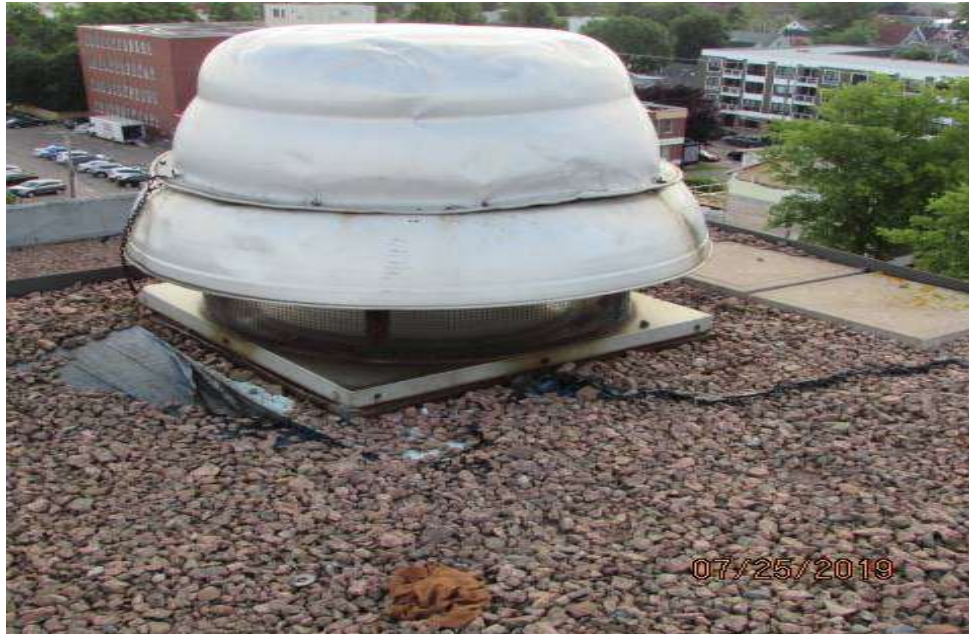
Ventilation unit in corner of roof.
