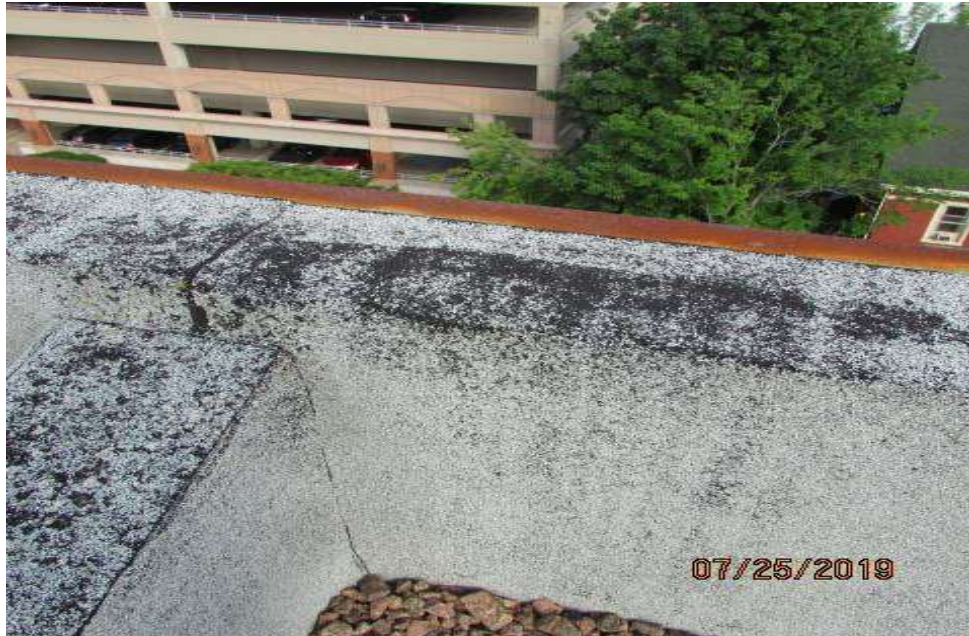
Severe granule loss on base flashing membrane.
