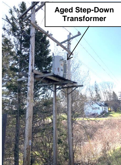
Aged Step-Down Transformer (1982 vintage)
