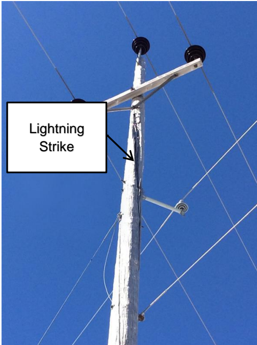
Damaged Pole (reduced pole strength)
