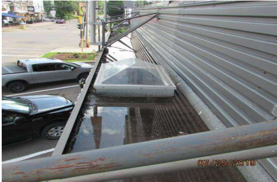
Ponding water on roof surface.
