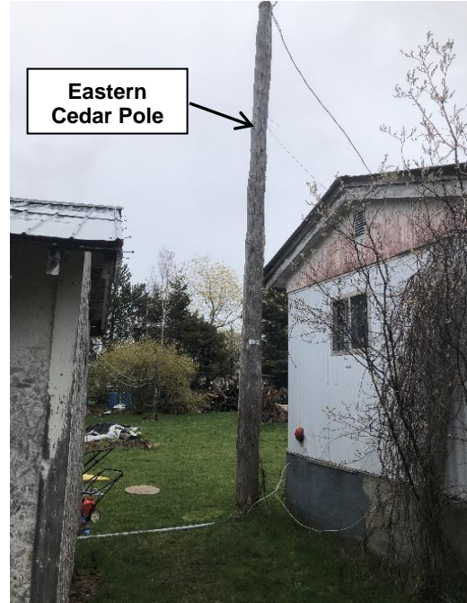
Aged and Deteriorated Pole
