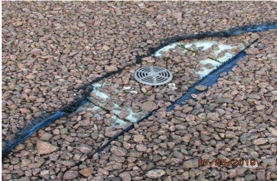
Fabric has been displaced on roof. This allows ballast to get down between insulation and roof membrane. This can damage the membrane.
