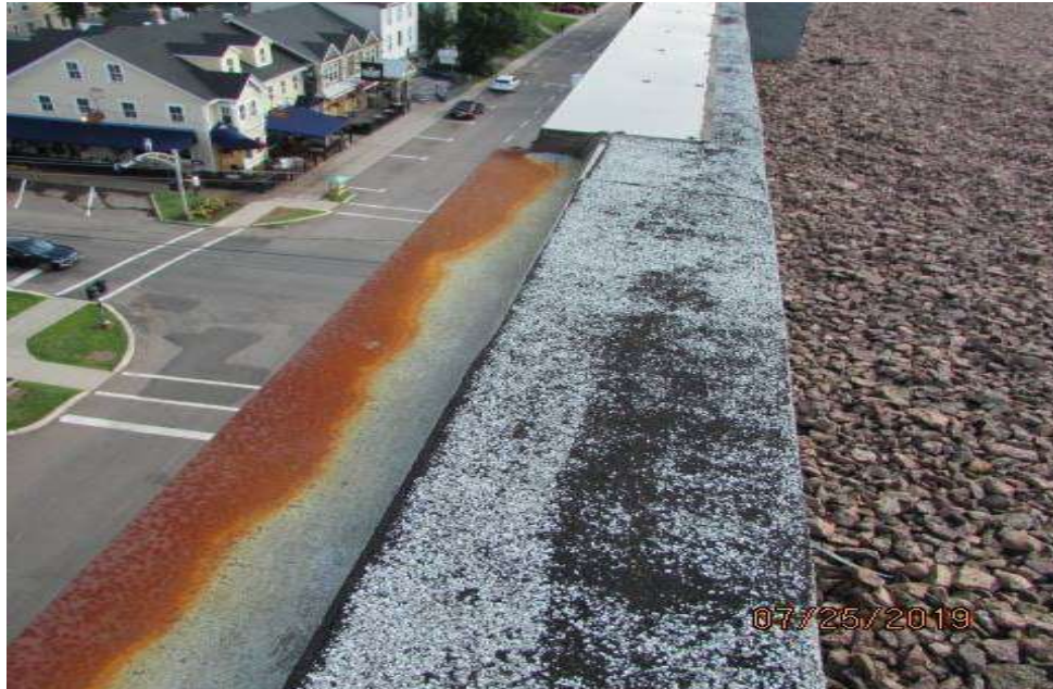
Severe granule loss on base flashing membrane.
