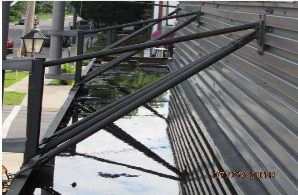
Excessive amount of water on roof surface.
