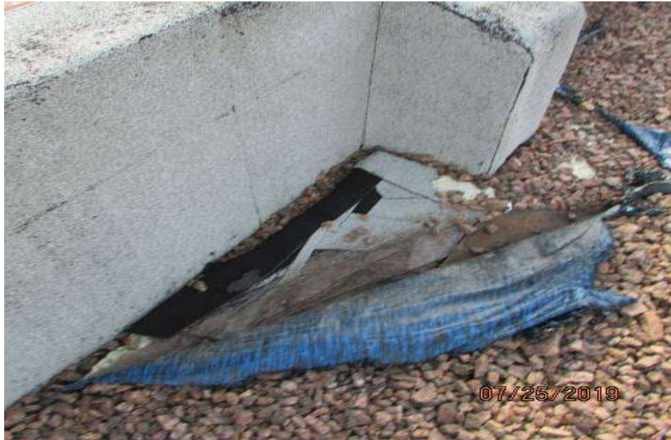
Repairs made to base flashing sub-standard.
