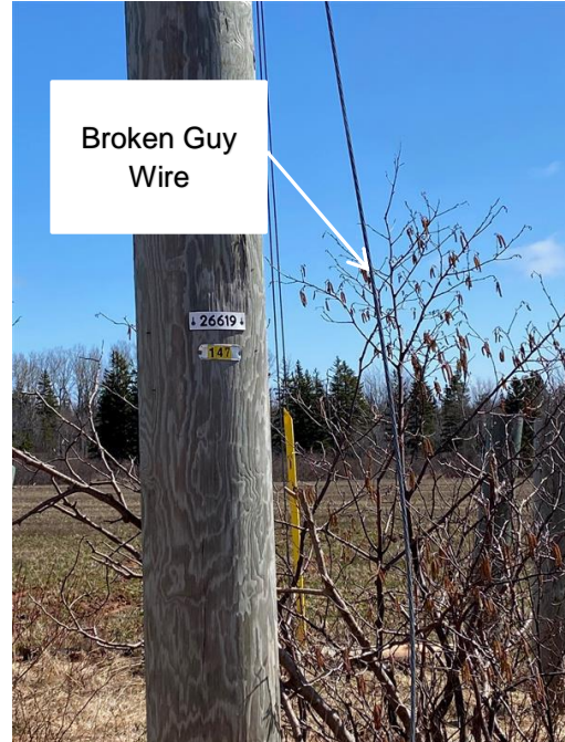
Damaged Pole Support (safety hazard)
