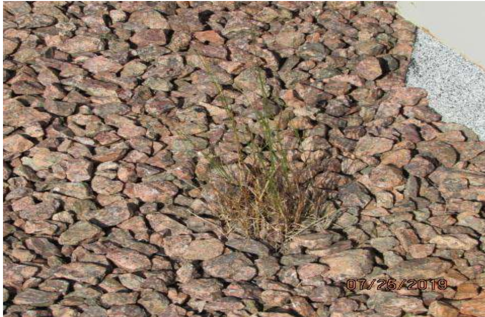
Vegetation growth on roof surface,
