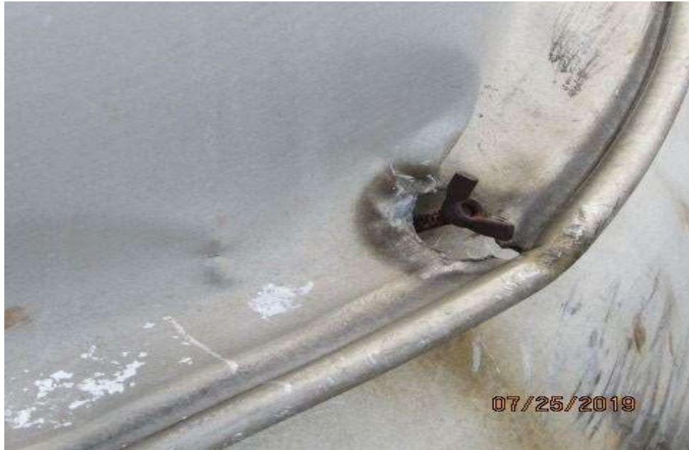
Fasteners for securing the cap of the vent hood appear to be in poor condition.
