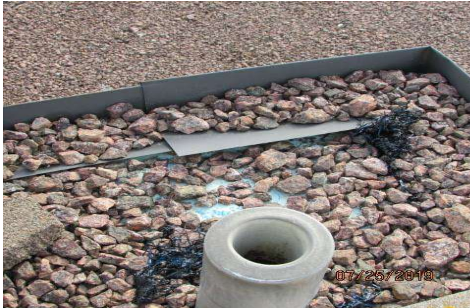
View of perimeter metal counterflashing. It appears loose with ballast underneath.
