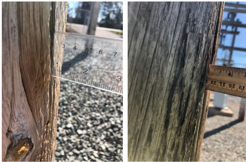
Poles are split with depths of 1 inch (left) and 3 inches (right).
