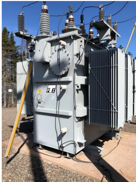
The transformers in service at Crossroads do not currently have oil containment systems. Oil containment systems will be installed for the new transformers as part of the Crossroads Substation rebuild.
