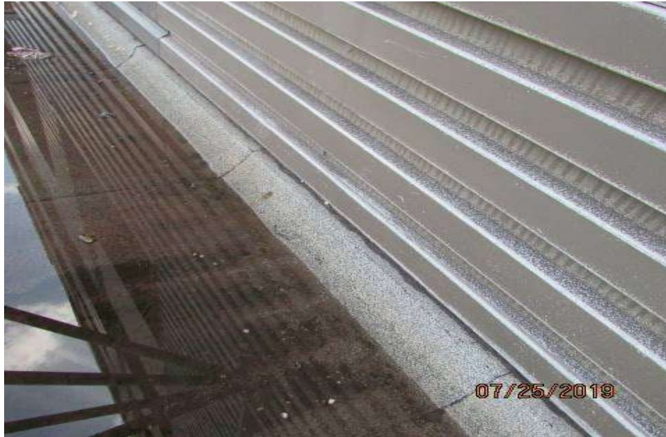
Excessive amount of water on roof surface.
