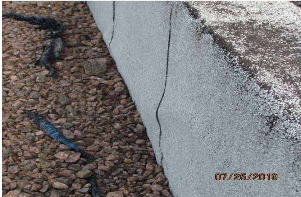
Loose base flashing membrane at wall parapet.
