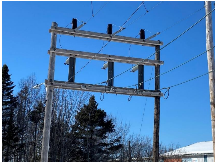
The mobile bay is aged and is not compatible with Maritime Electric's newest mobile transformer (due to the bushing locations on the mobile transformer).
