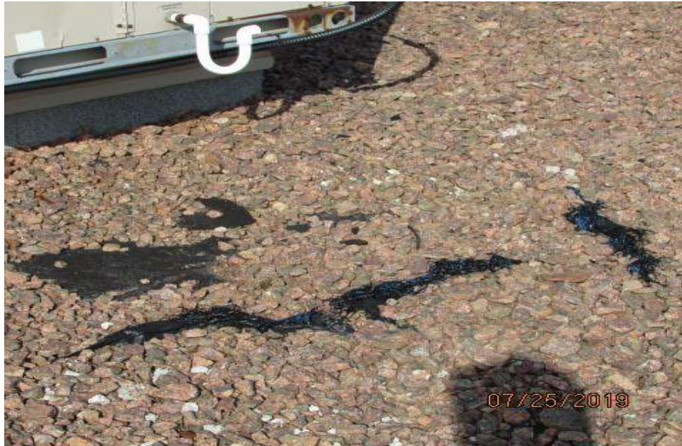
Ballast is displaced on roof surface. The scrim is exposed.
