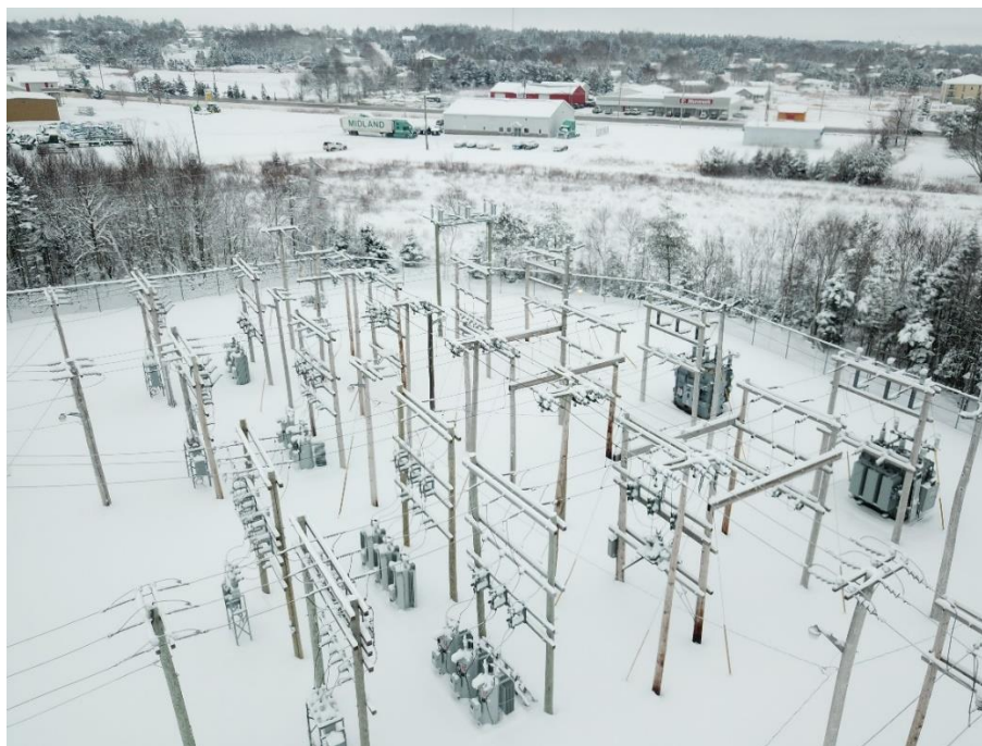
Figure 3: Crossroads Substation, Stratford, PE
