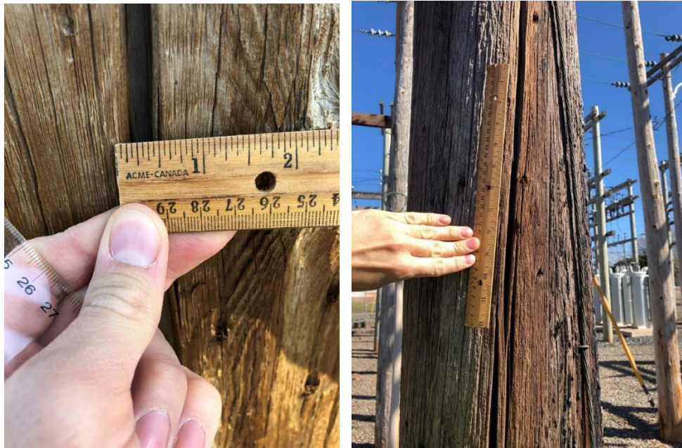
This pole split has a width of 0.50 inches (left) and a length of over 1 foot (right).
