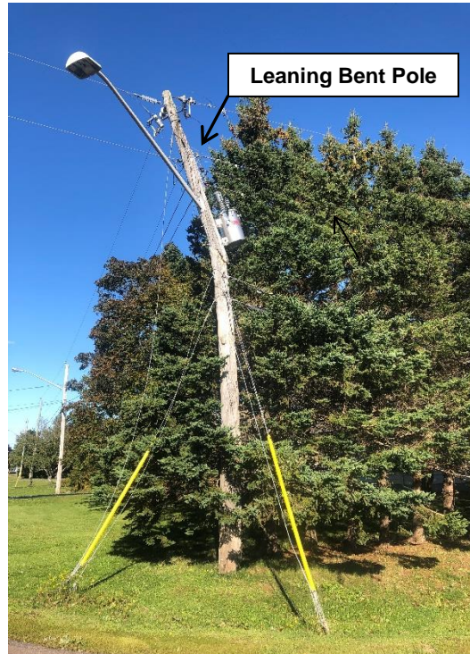
Damaged Pole (safety hazard)
