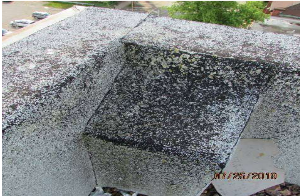
Severe granule loss on base flashing membrane.
