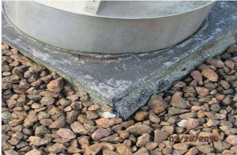
Base flashing membrane at base of stack in poor condition.
