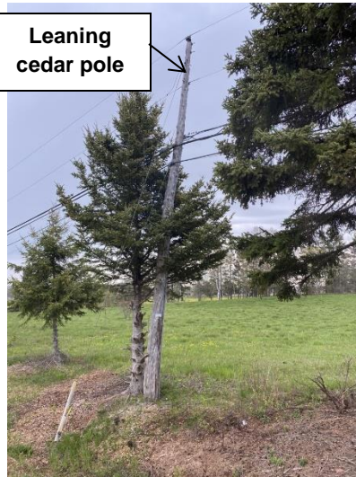
Leaning Eastern Cedar Poles
