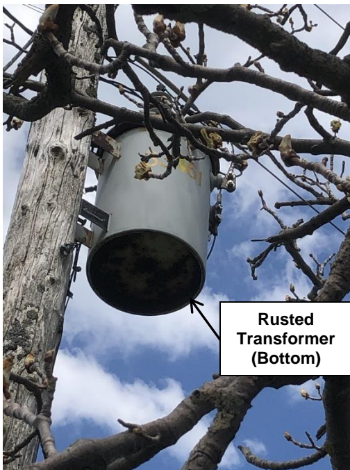
Deteriorated Equipment (oil spill risk)
