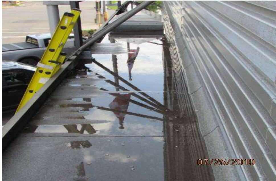
Ponding water on roof surface.
