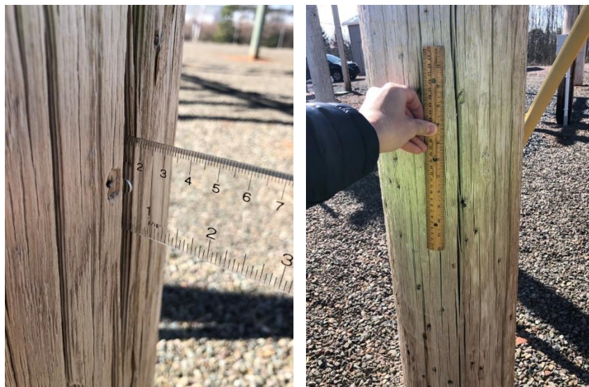
This pole split has a depth of 0.75 inches (left) and a length of over 1 foot (right).
