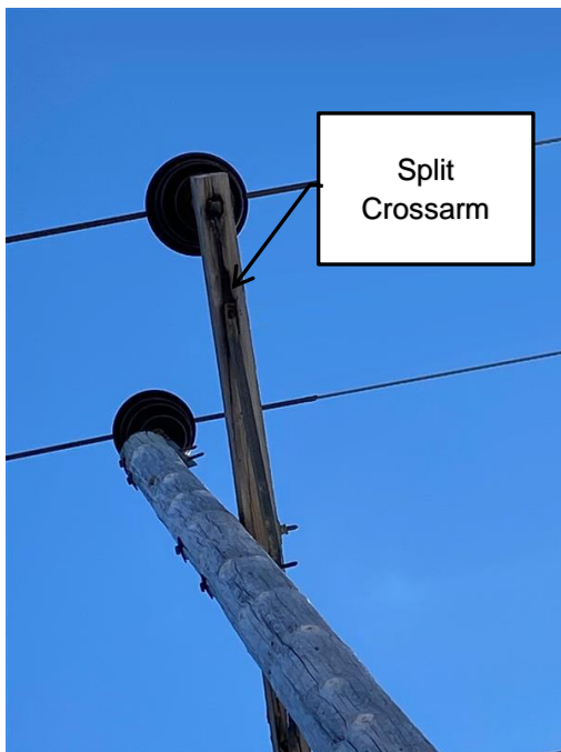
Deteriorated Crossarm (safety hazard)
