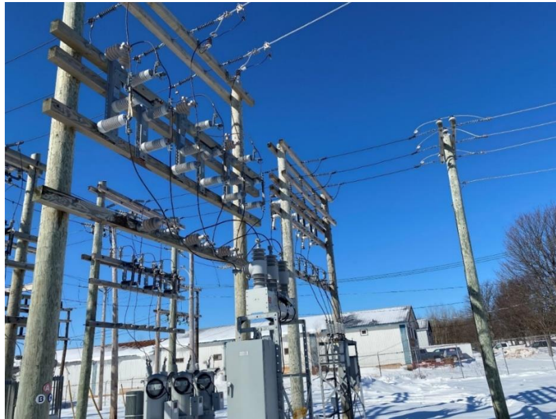
Safety clearances within the station do not meeting current standards.
