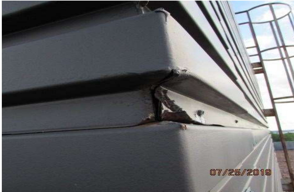
Damaged outside corner of metal cladding to penthouse.
