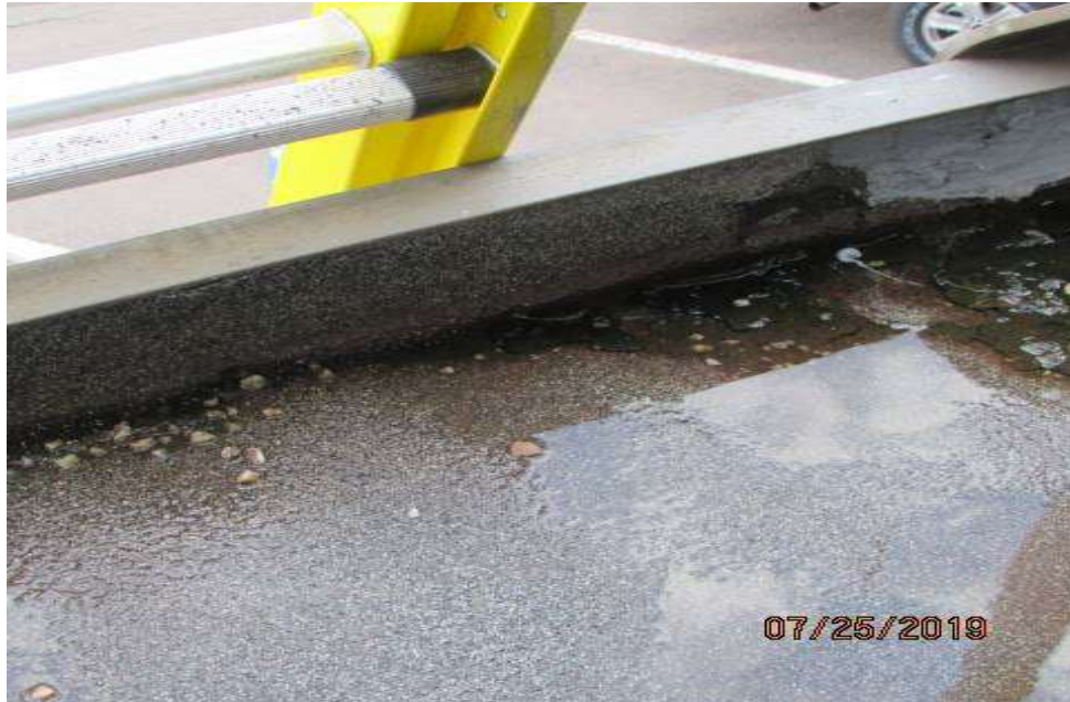
Area of deteriorated decking and insulation. Water setting inside.
