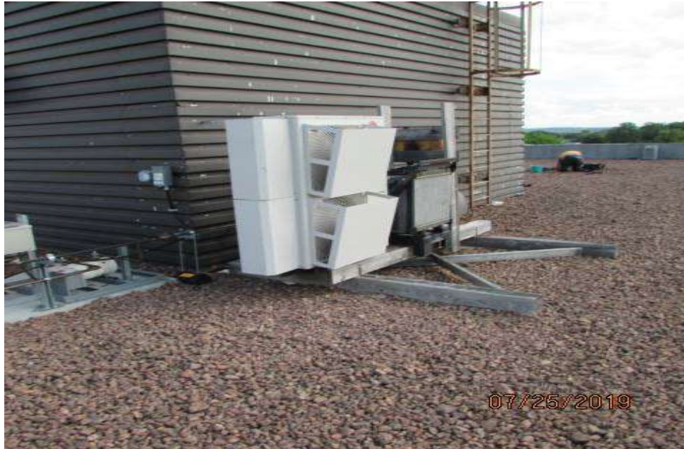
View of roof top units on roof.
