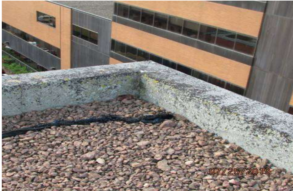
Severe granule loss on base flashing membrane.
