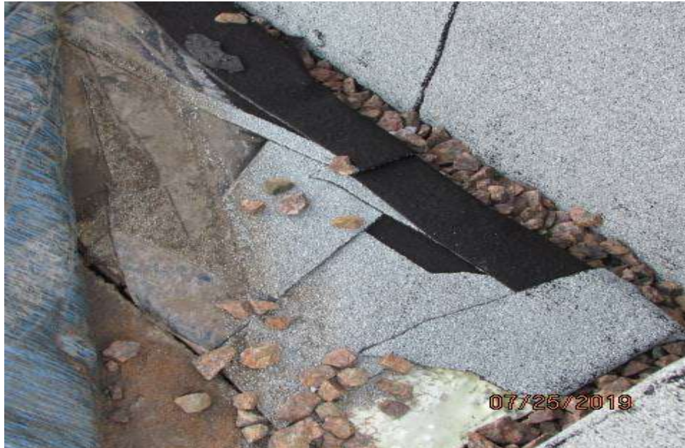
Repairs made to base flashing sub-standard.
