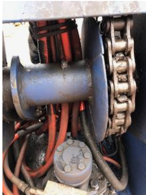
Truck 12-12-58 Condition of elevator drive chain & hoses
